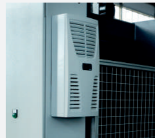
Electrical Cabinet Cooling System
